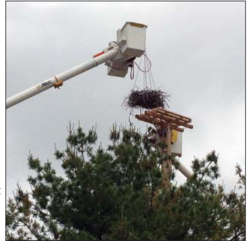
JCP&L crew moves an Osprey nest in Oceanport off a power pole to a new, safer platform.
